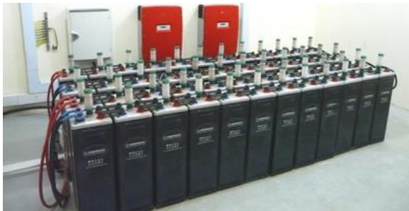
Deep cycle storage batteries at the Oryx Center Photo: May Yoke Taylor
